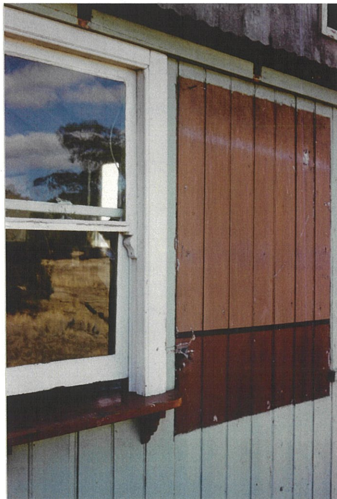
Figure 4.1 Wal Wal: detail view showing use of Terra Cotta and Mid Brown. (A. Ward)
